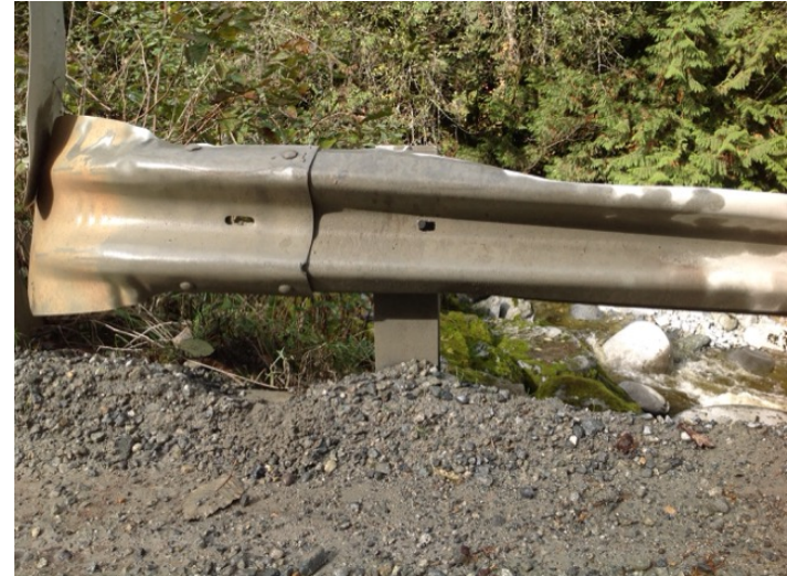
guardrail not bolted to post upstream right approach
