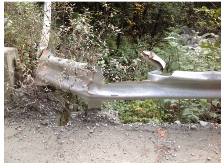
guardrail damage left downstream approach
